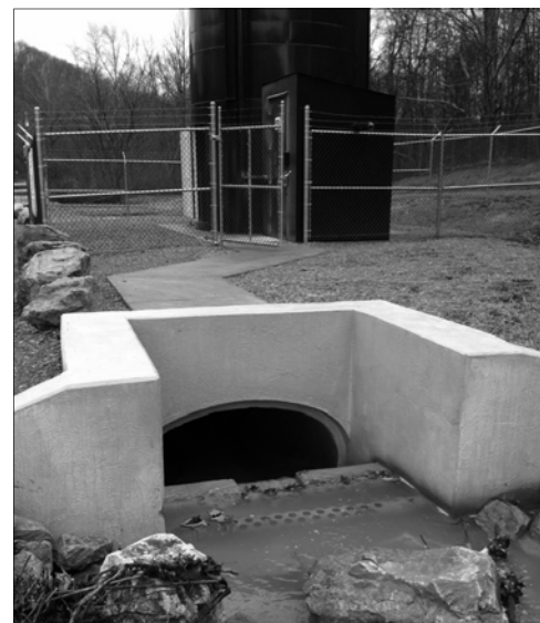
Thomas Fork Doser located on Bailey Run Road helps neutralize acid-mine drainage by depositing limestone into the creek.
